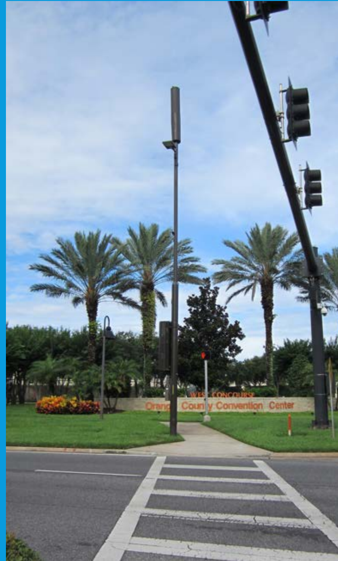
Camouflaged Antenna on Streetlight with Radios in Pole-Mounted Shroud
