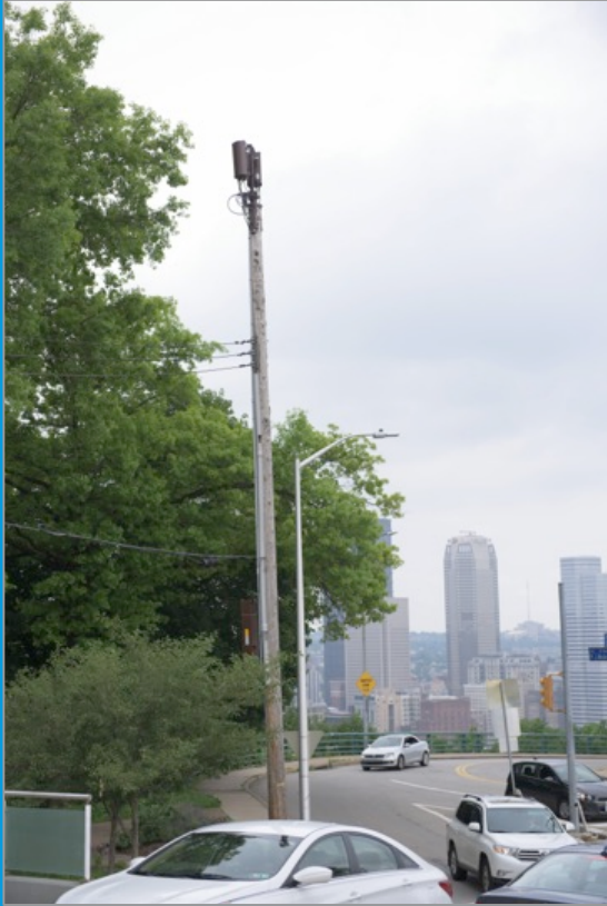
Wood utility pole
