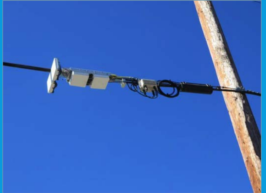
Strand mount on utility cable
