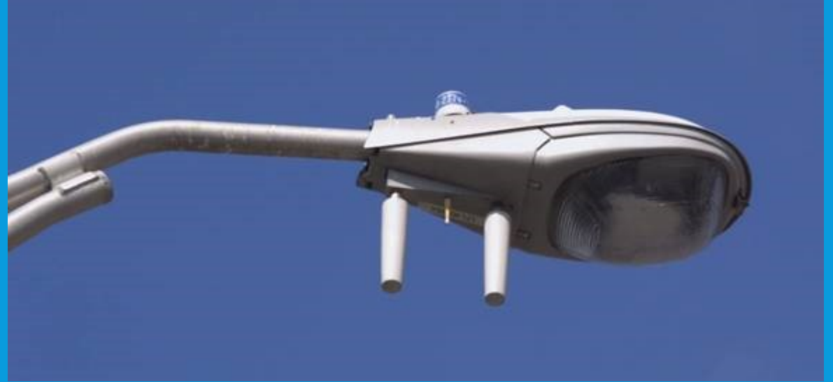
Equipment on lamp of streetlight
