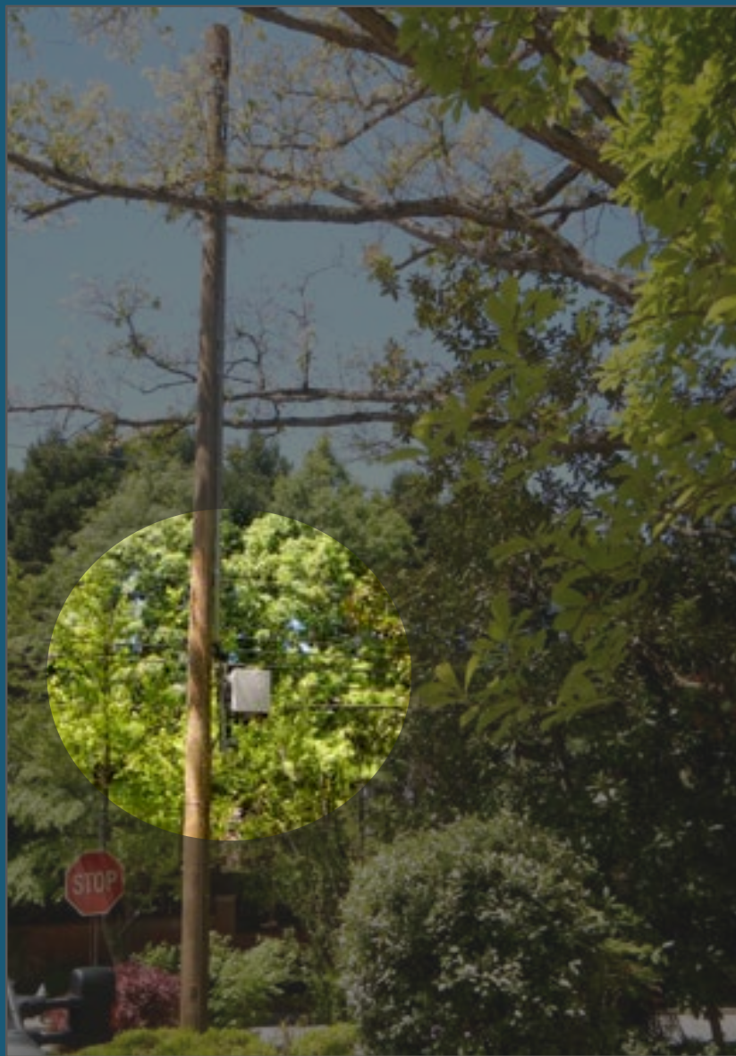
Wooden pole with equipment shroud
